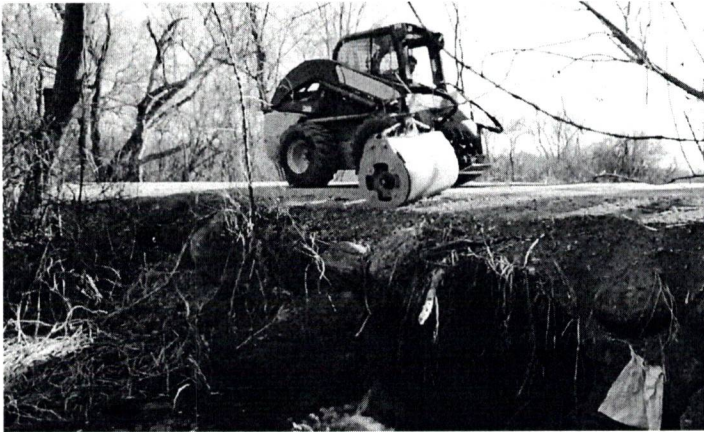
Offset feature allows operator to stay on the road while rolling and compacting shoulders and ditches.
